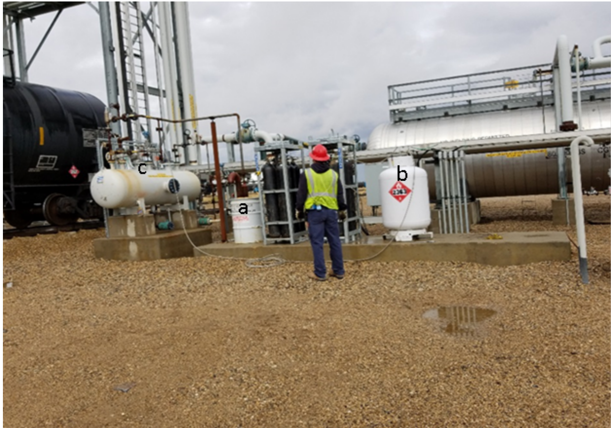
Figure 5. A) Photograph of the work area where the ethyl mercaptan tank transfer was performed. a) Vent trap for nurse and metering tank. b) Nurse tank. c) Metering tank
